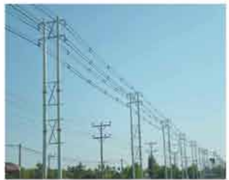
33 KV DOUBLE CIRCUIT O/H LINE @ KYANSISMINN
