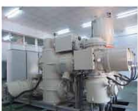
66/11 KV, 2 X 30 MVA GIS SUBSTATION @ YADANA
