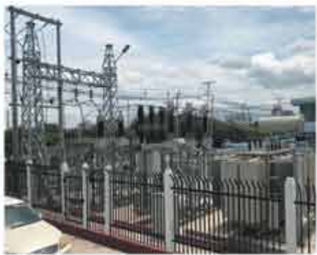
33/11 KV, 10MVA SUBSTATION @ MYAYEENANDAR
