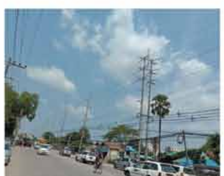
66 KV DOUBLE CIRCUIT O/H LINE @ FORTUNE PLAZA
